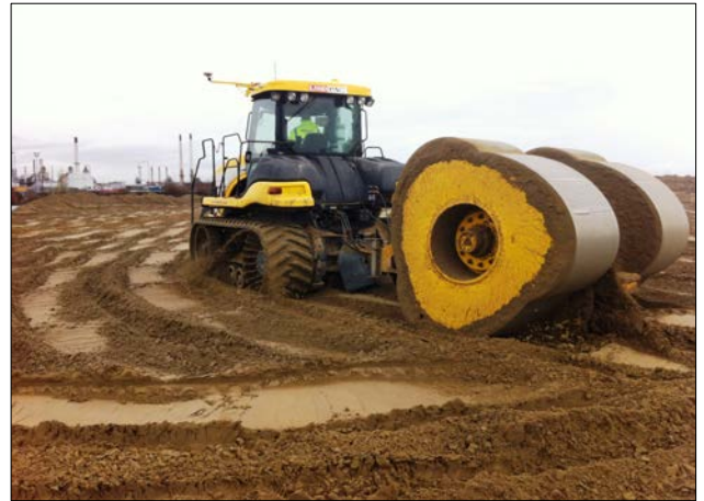
Figure 5: HEIC on dredged Sand materials at the London Gateway Container Terminal, UK
